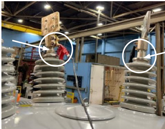
Red Lead (H1) connection to Load (L) Bushing
