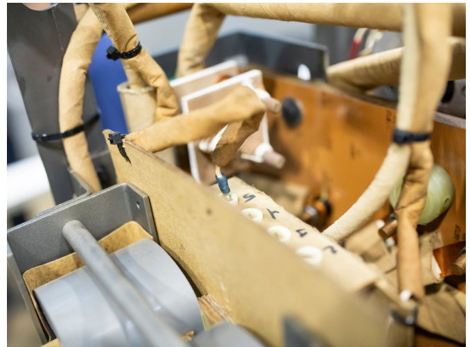
Figure 8. Potential Transformer Terminal Board Hand-Hole Opening View
