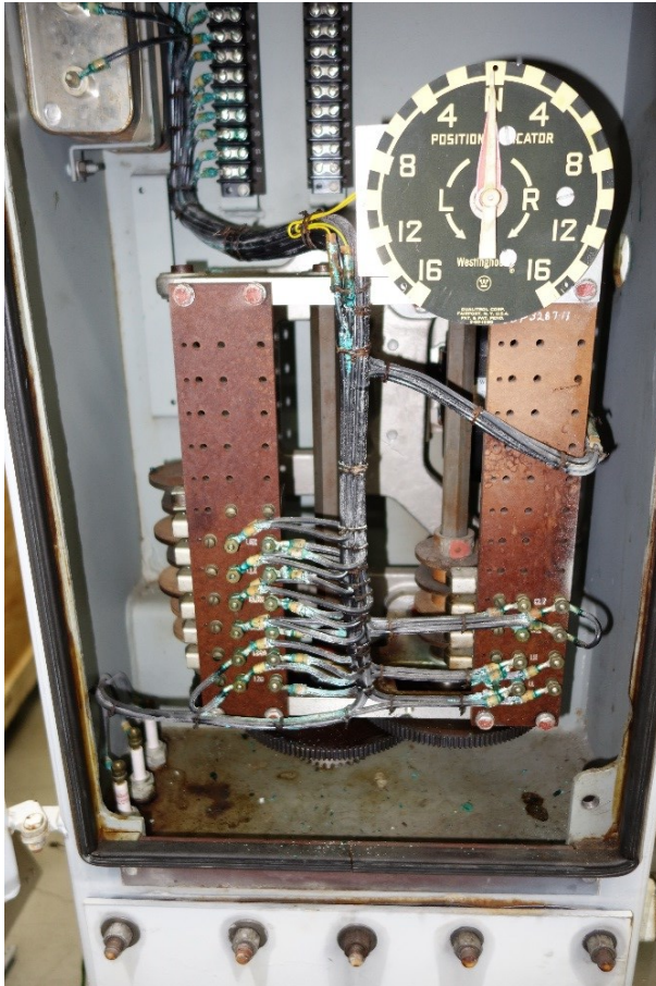
Corrosion and Wiring Insulation Degradation in Cam Switch Compartment
