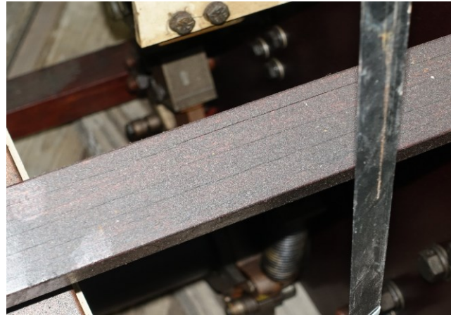
Cracks in Phase Board Insulation
