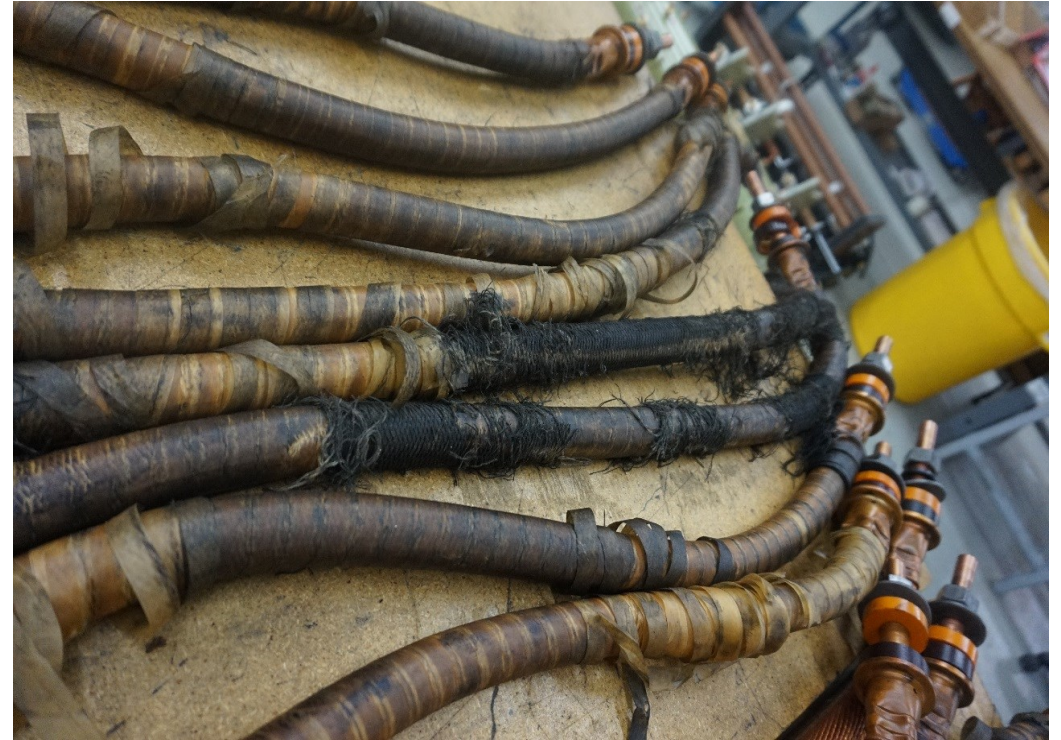
Tap Leads with Insulation Damage & Heating
