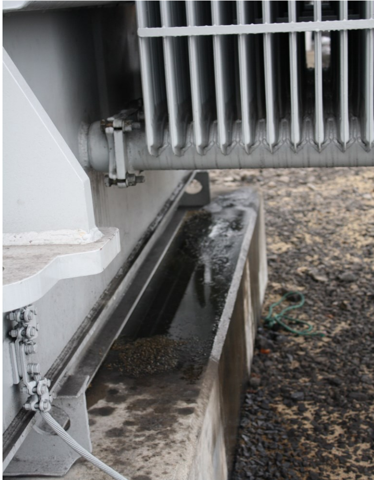
Blocked Cooling Fins
