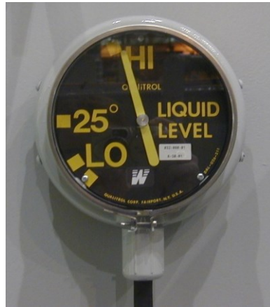
Typical tank mounted liquid level gauge
