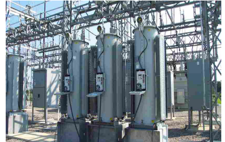
3ph bank at substation bus
